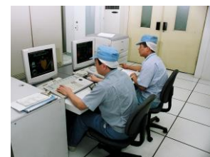
Central control room
